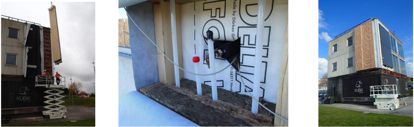
Figure.5: The demonstrator at the Kubik building, based on the installation of the modules, fitting the services and final finishing.
